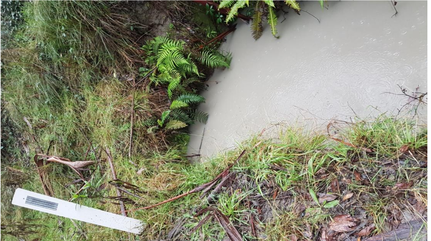
Another almost fully blocked culvert entry under Snobs Creek Rd (11/4)
