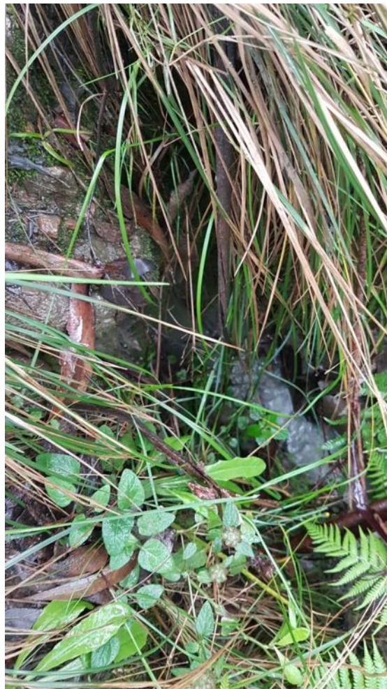
Evidence of low outflow from culvert (above)
