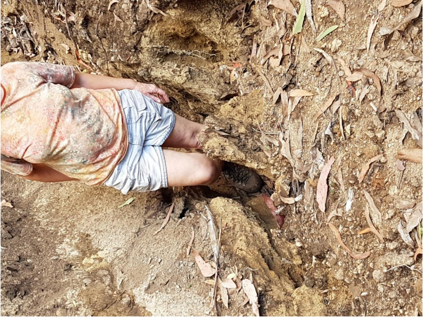
Gully in road (17/3)
